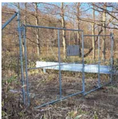
△有害獣侵入防止柵
